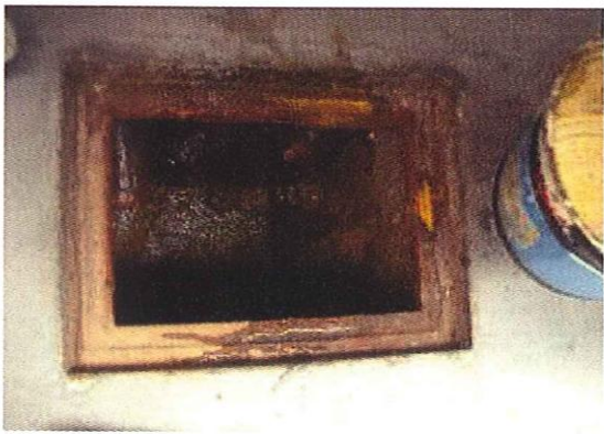
Dye test of manhole near 2/F East Terrace.
