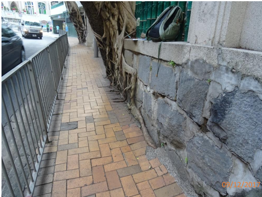
Severe cracks on the retaining structure
