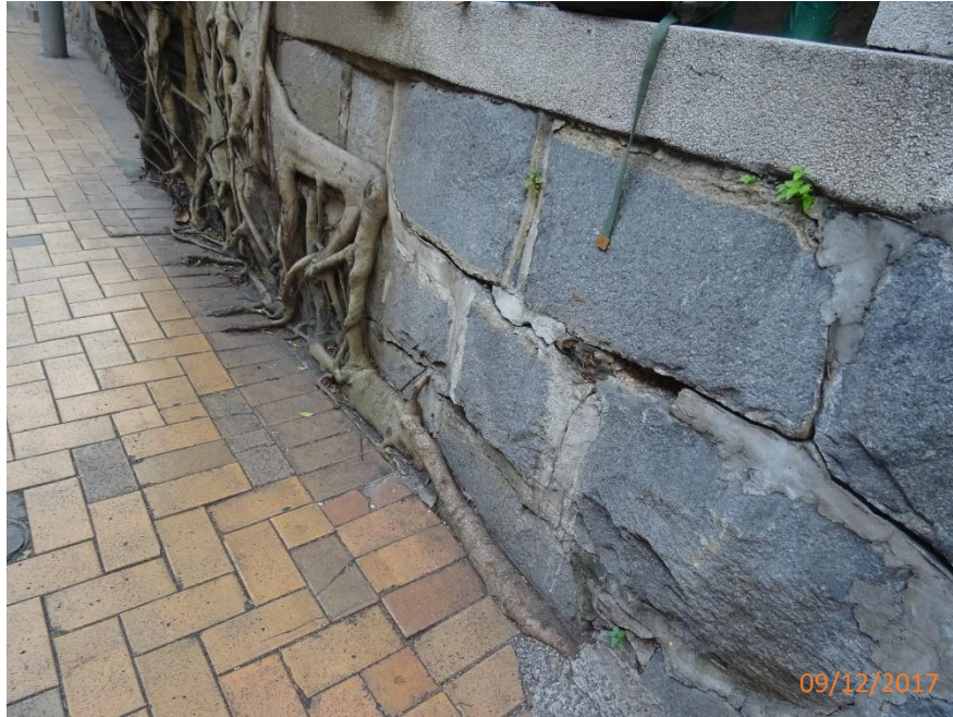
Close-up of the cracks
