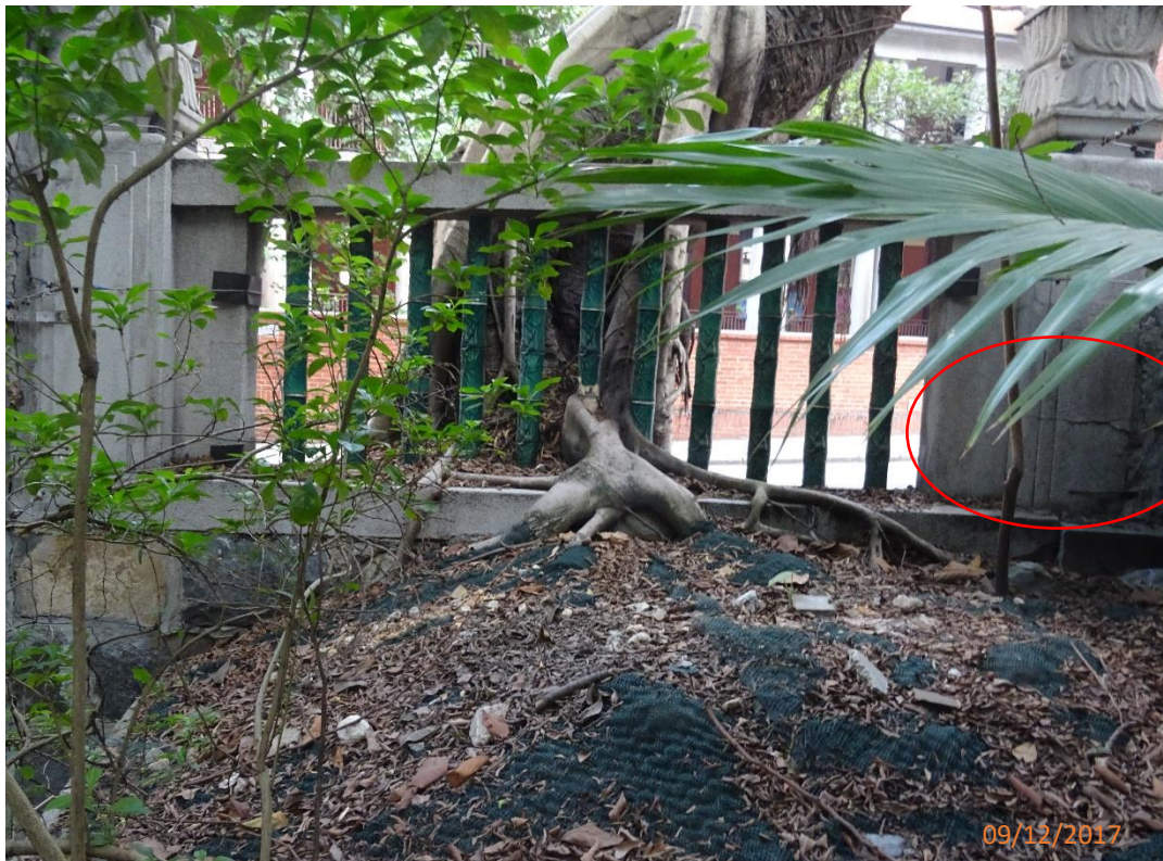
Tension side of the tree anchor into the slope planter. Cracks on retaining wall.
