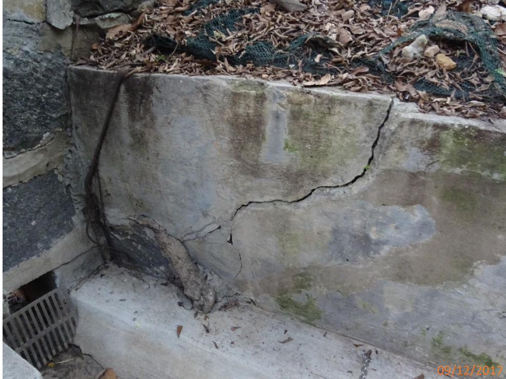
Cracks on the planter behind the tree
