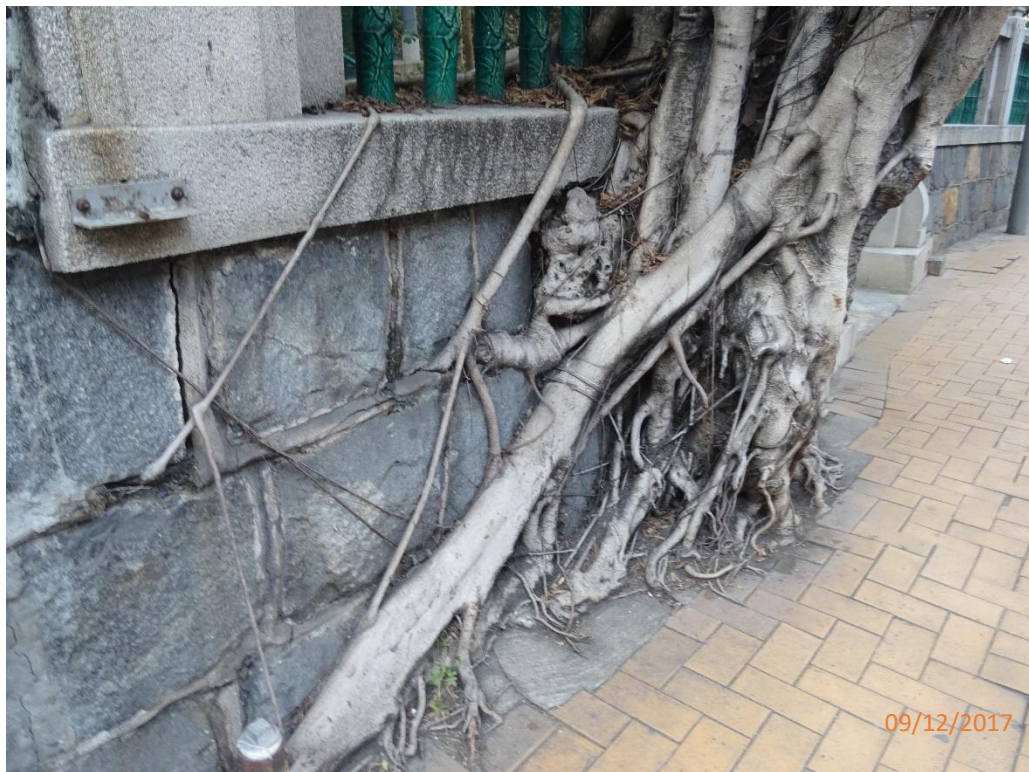
Cracks on the retaining structure
