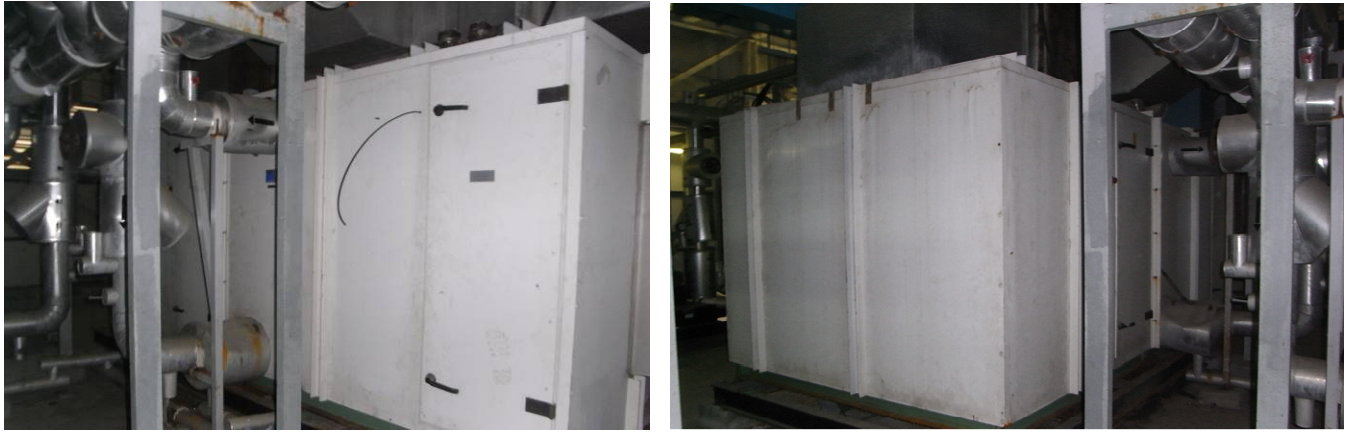
鮮風櫃 (Air Handling Unit)
