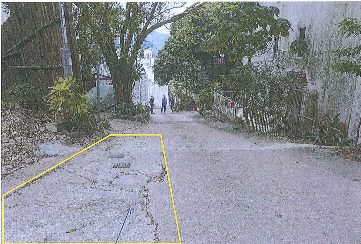
View 2 (擬維修的破損路面)
