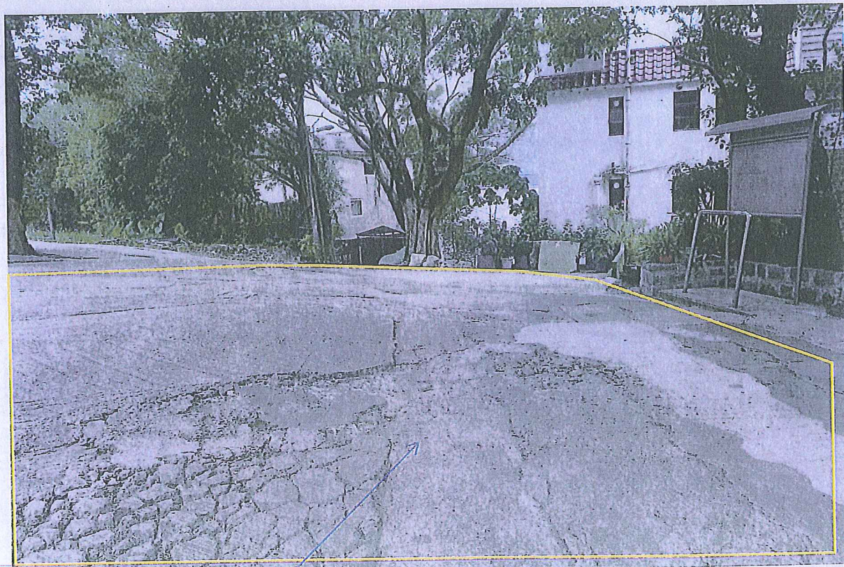
View 1 (擬維修的破損路面)
